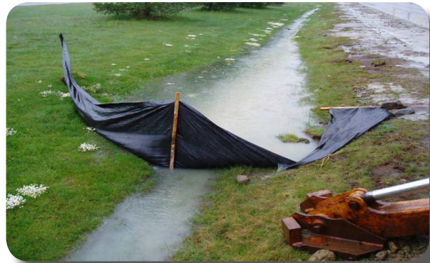
Poor erosion control can add sediment.
